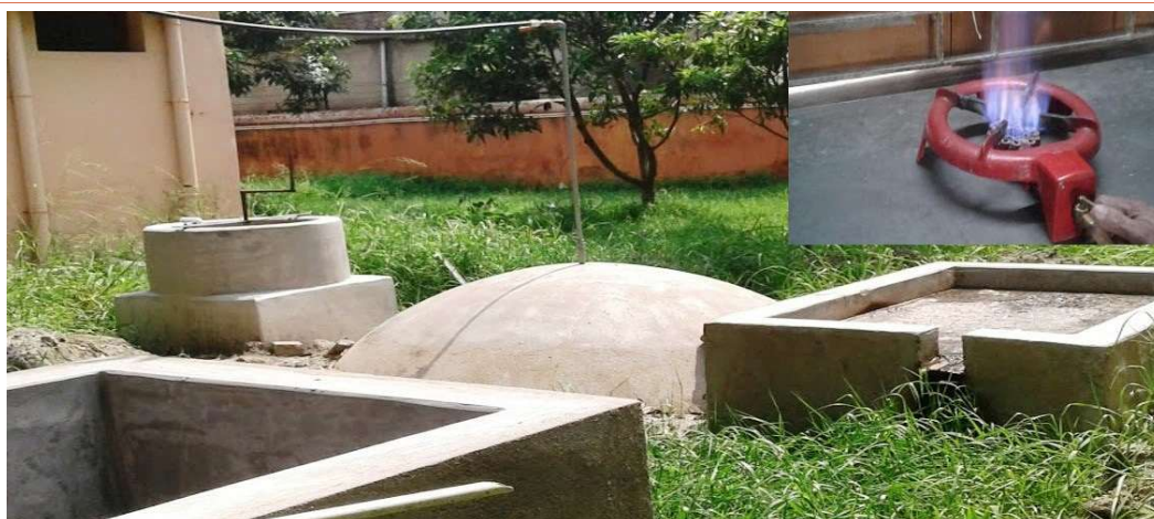
A biogas plant from kitchen waste is installed at APC College, Madhyamgram, North 24 Parganas, by VIB.
